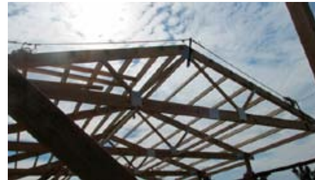
Figure 3. Vertical lifeline installed on a truss. Note the rope grab on the left side.
