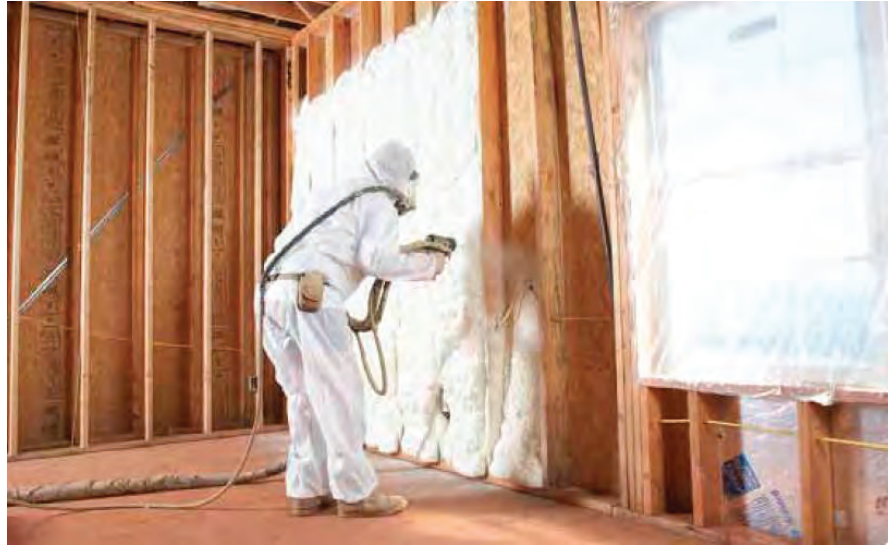
FIGURE 2. A typical spray polyurethane foam insulation application. The worker applying SPF needs complete personal protective equipment, including an air respirator, eye protection, chemical-resistant clothing and chemical-resistant gloves.
