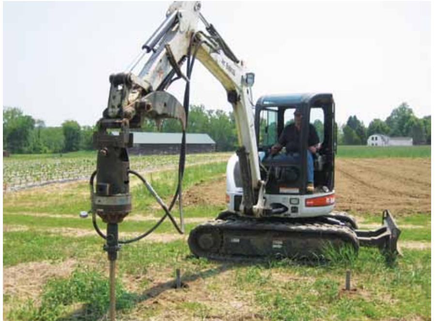
FIGURE 15. A specialized mini-excavator attachment for screw pile installation. (Source: Frame Building News )
