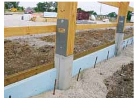
FIGURE 12. Precast concrete piers with a grade beam (Source: Robert Meyer). A detail showing precast concrete piers with a grade beam or “ribbon” may be downloaded from http://bit.ly/1BMdgNG .
