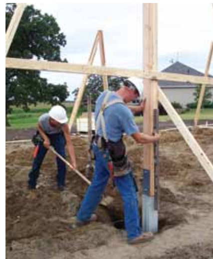
FIGURE 8. Precast concrete piers attached to wood posts and plumbed like a wood post set in soil. (Source: Robert Meyer)
