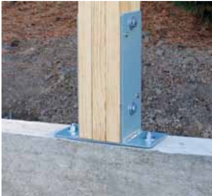
FIGURE 13. Illustration of a post anchored to a concrete basement wall with a drill-set bracket. (Source: Brandon Meyer)
