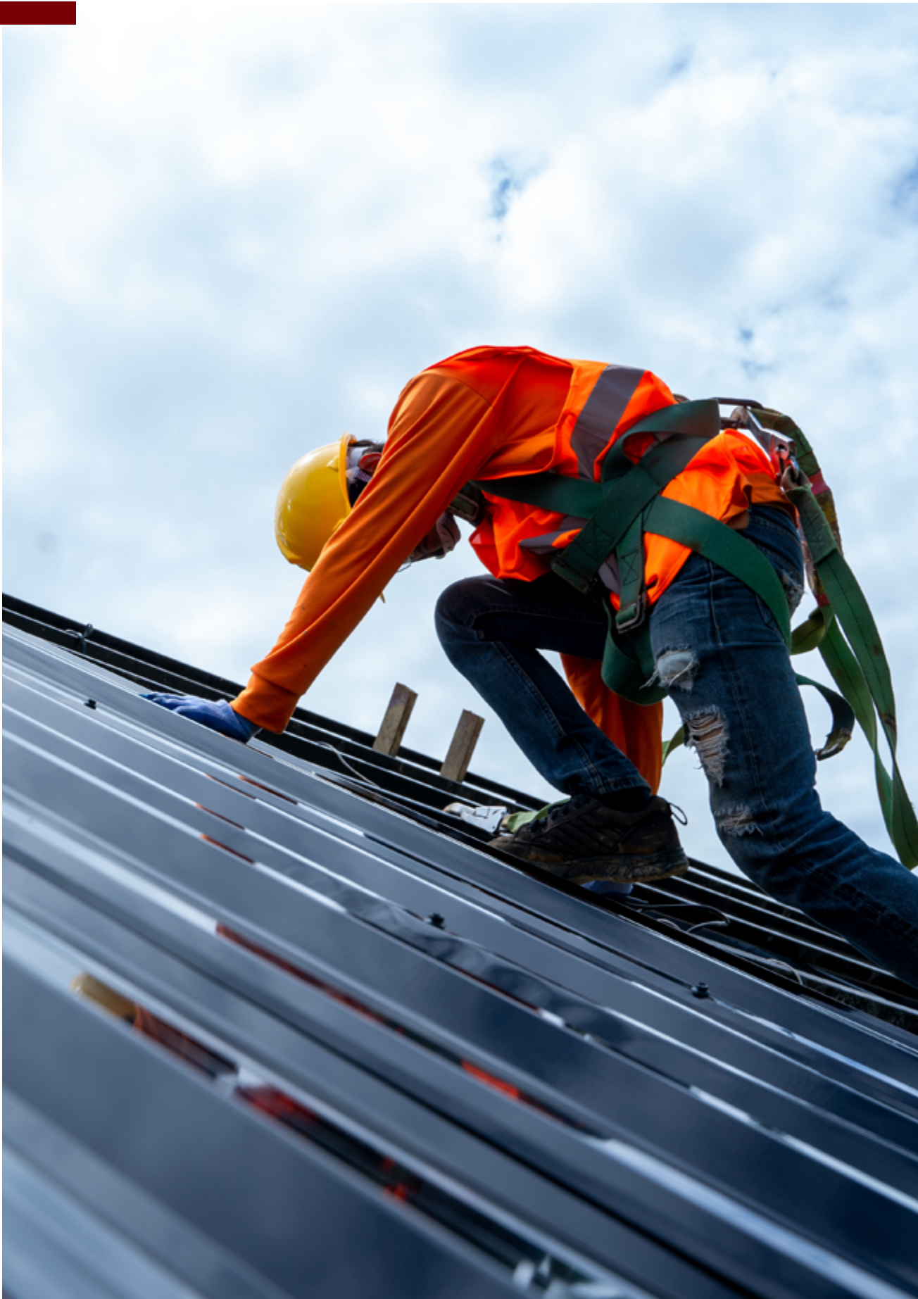
While any employee is inspecting a walking/working surface for its integrity, that employee must use a personal fall arrest system.
