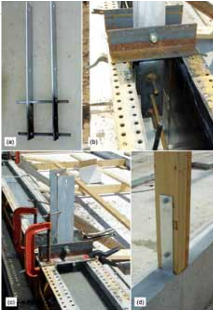
Figure 20. Post-to-concrete wall connection with straight side plates: (a) plate width fixed with two short rebar; (b) top of wall reinforced with horizontal rebar passed through plates; (c) angles and clamps used to fix bracket in place during concrete placement; (d) finished connection.
