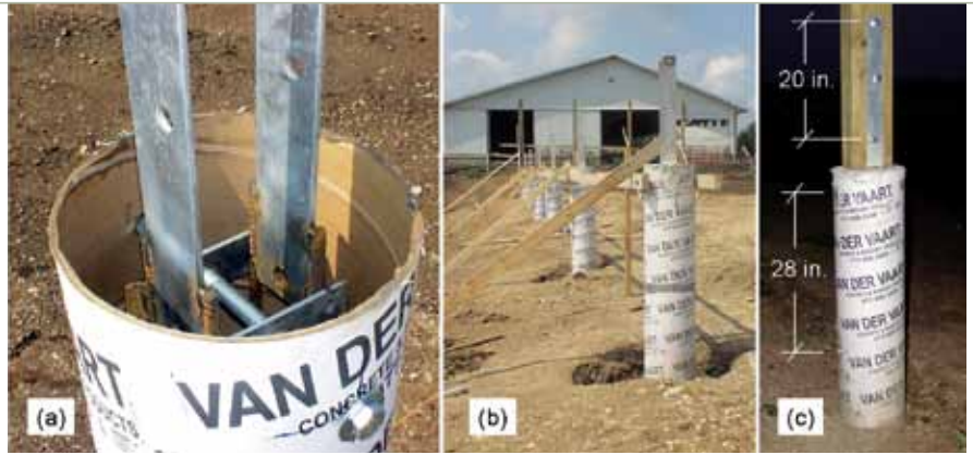
Figure 21. Post-to-concrete pier connection featuring straight side plates welded to steel reinforcing bars. Threaded rod with coupler nuts and bolts used to: (a) fixed bracket into place, (b) attach temporary wood braces to pier, and (3) provide anchoring points (at a 28 inch spacing) for steel partitions and gates.
