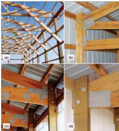
Figure 11. Four different post-to-truss connections: (a) regular heel truss with kneebrace, (b) raised heel truss, (c) deep heel truss, and (d) regular heel truss without kneebrace.
