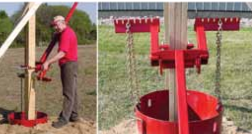
Figure 4. Lever is rested on quick-attach fulcrum and then chained to the posthole installation shield.
