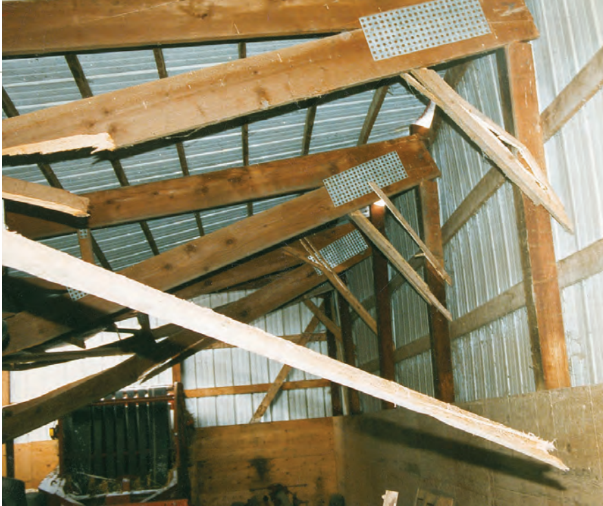
Here the knee braces slipped relative to the truss chord and post, and eventually failed as the roof failed under the snow load.
