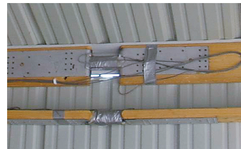
Figure 9. – Frame force monitoring links (FFML) mounted in an eave strut and top girt.
