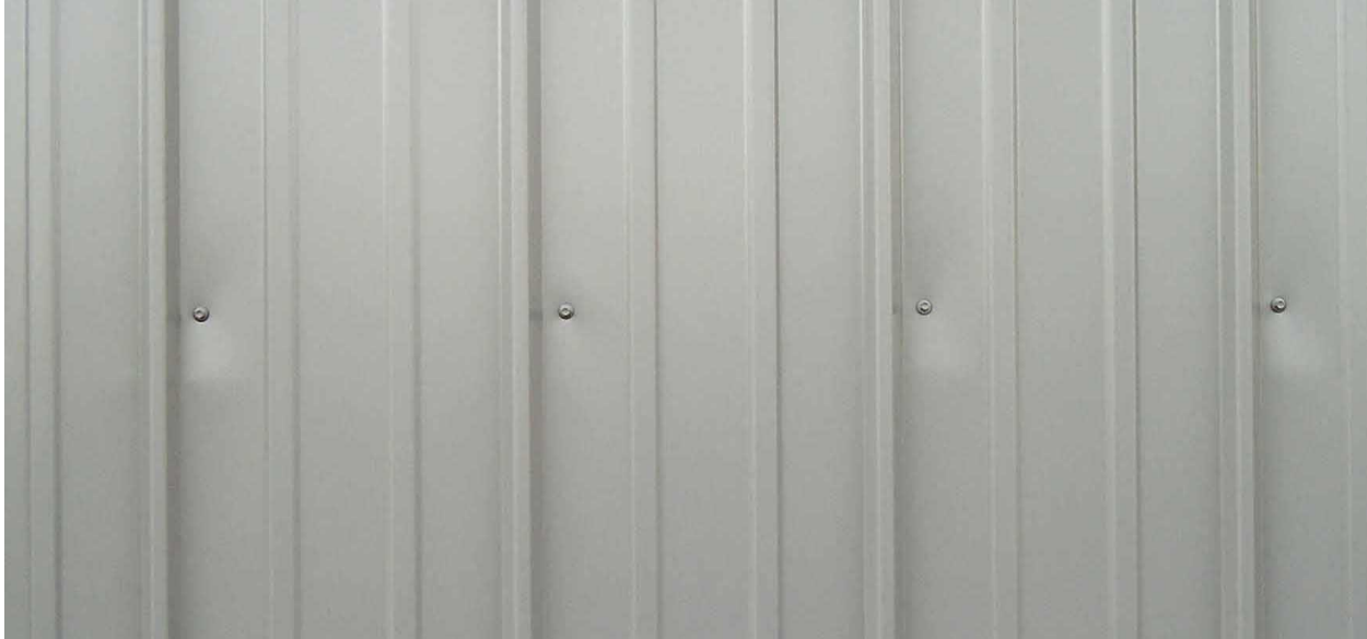
Figure 12 - Panel attachment to a cupped girt results in noticeable depressions around fasteners.
