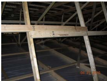
New lateral brace connection
