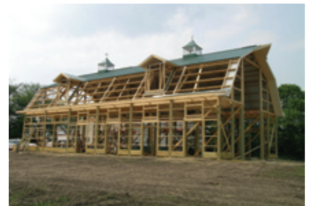
ABOVE: The McIntosh project, in Watertown, Minn., is a post-frame construction by Lester Buildings.
